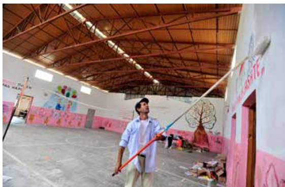
Rehabilitation work at the Së Bashku school in Gjirokastër — painting the interior of the school, which also serves as a sport hall.
